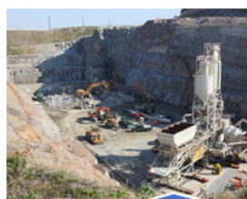
Concrete Batch Plants
