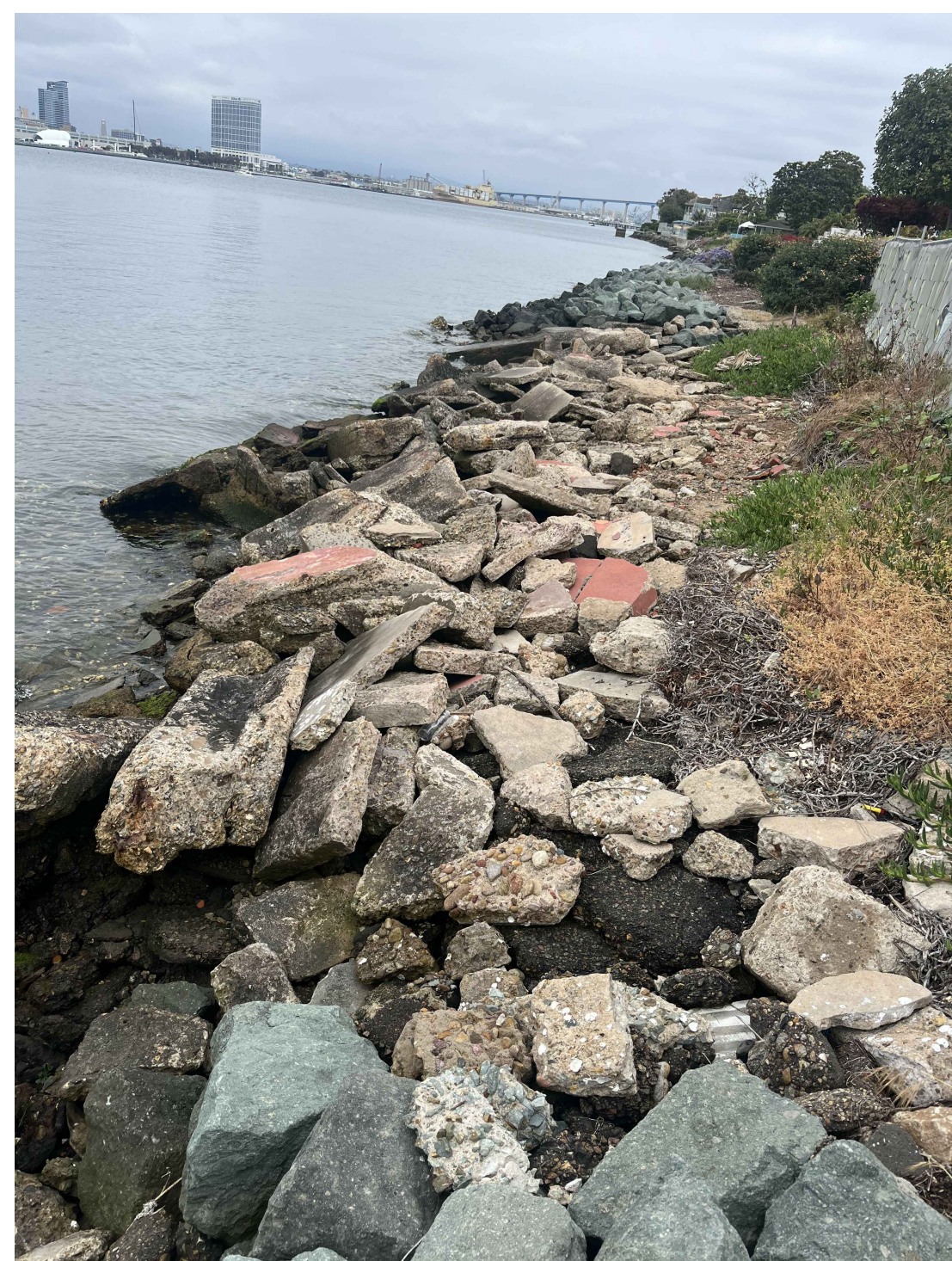
PHOTO 2, LOOKING SOUTHEAST FROM PROPERTY LINE BETWEEN 409 AND 407 1ST STREET. NOTE ALL EXISTING REVETMENT MATERIALS FRONTING 409 1ST STREET CONSIST OF BROKEN CONCRETE DEBRIS, ALL OF WHICH IS TO BE REMOVED AND DISPOSED OFFSITE. NEW REVETMENT STONE TO BE PLACED TO THE SAME GRADES AS THE ROCK REVETMENT ON THE ADJACENT PARCEL TO THE SOUTHEAST.
